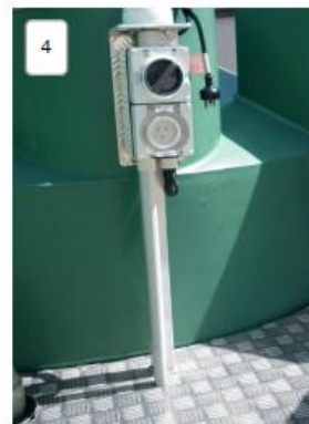
Transfer Pump Power Point
