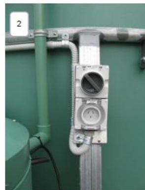
Grease Trap Lifting Pump Power Point
