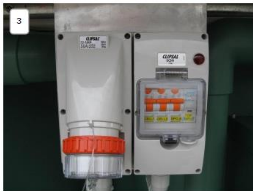
Mains Power Connection Point
